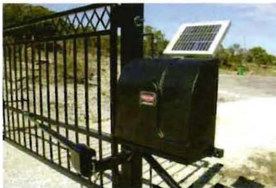
Rather than relying on electrical exhaust fans, why not consider sun light to power them where available. The same holds true with gate openers.
