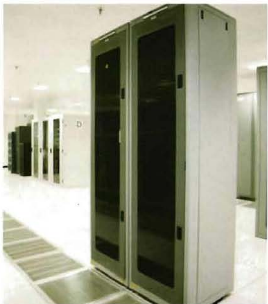
Use new energy efficient servers that have reduced heat generation to reduce power consumption.
