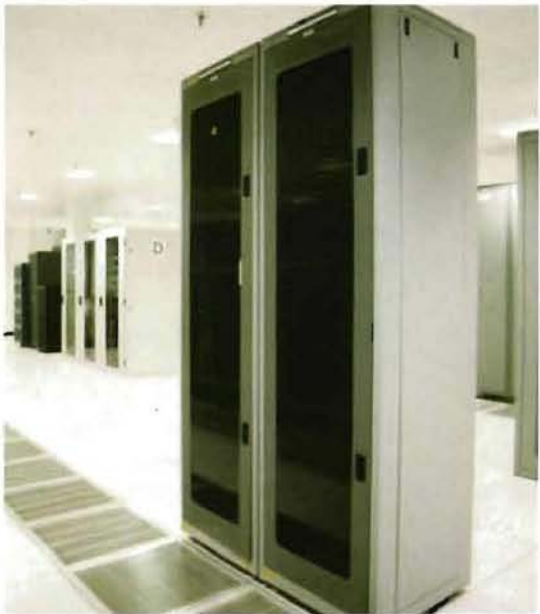
Use new energy efficient servers that have reduced heat generation to reduce power consumption.
